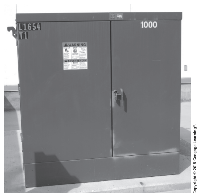
FIGURE 2-39 Pad-mounted transformers are generally contained in vaults.
