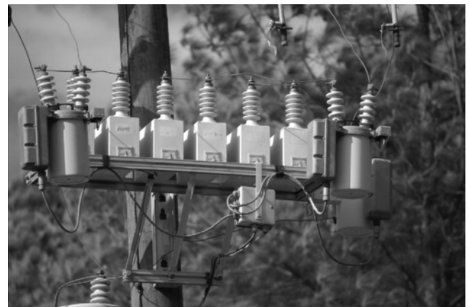
FIGURE 11-12 Capacitors used for power factor correction.
