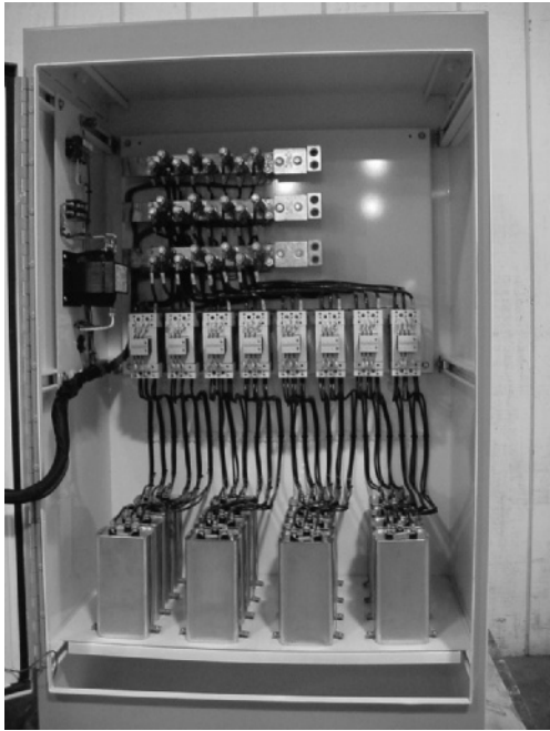
FIGURE 11-22 Capacitors used for power factor correction.
