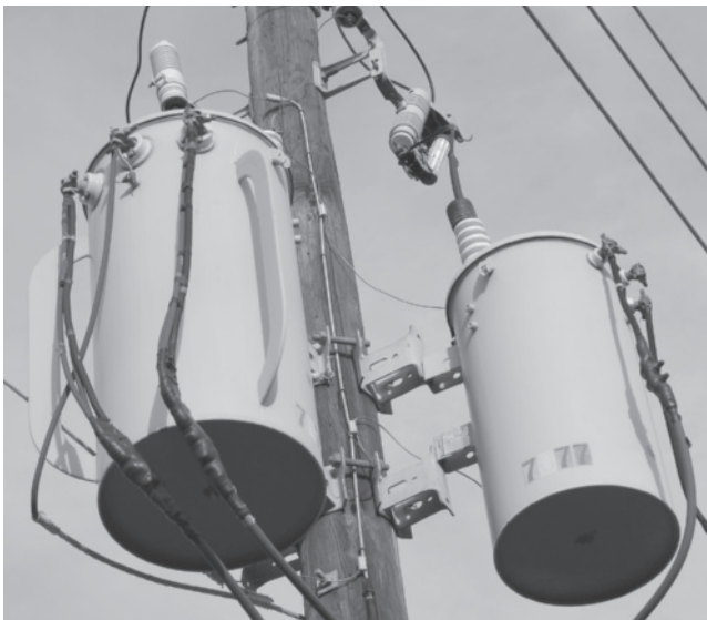
FIGURE 2-27 One transformer is larger than the other.
