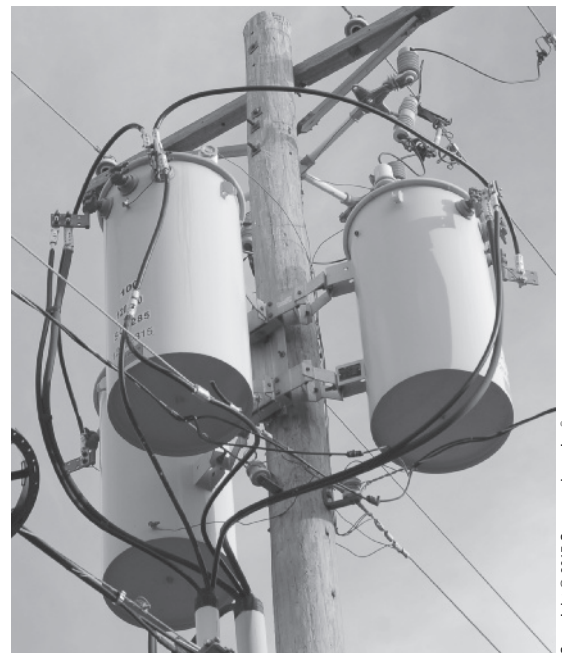
FIGURE 2-22 Single-phase transformers mounted on a pole and connected to form a 3-phase bank.
